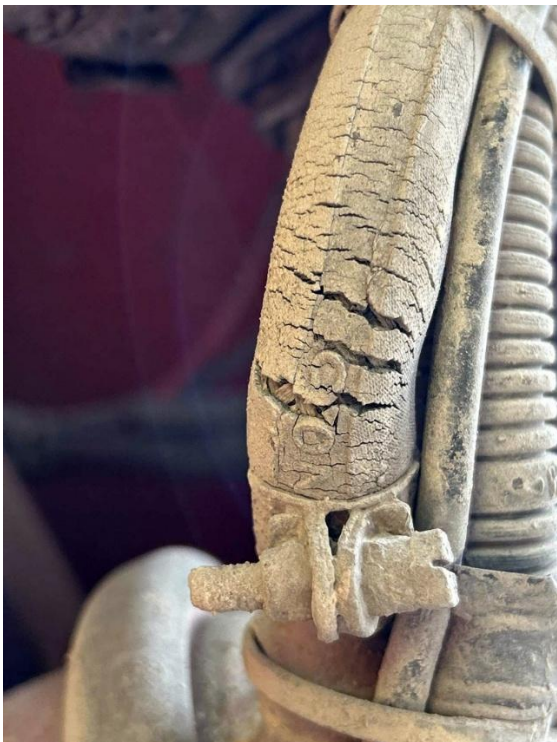
Figure 3: Worn and leaking pneumatic air line (M. M. Sanchez, 2026)
